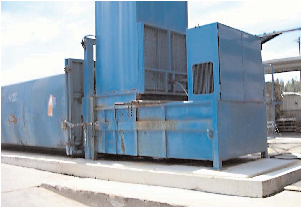
Compacting solid waste can help reduce transport costs and save on storage space.
