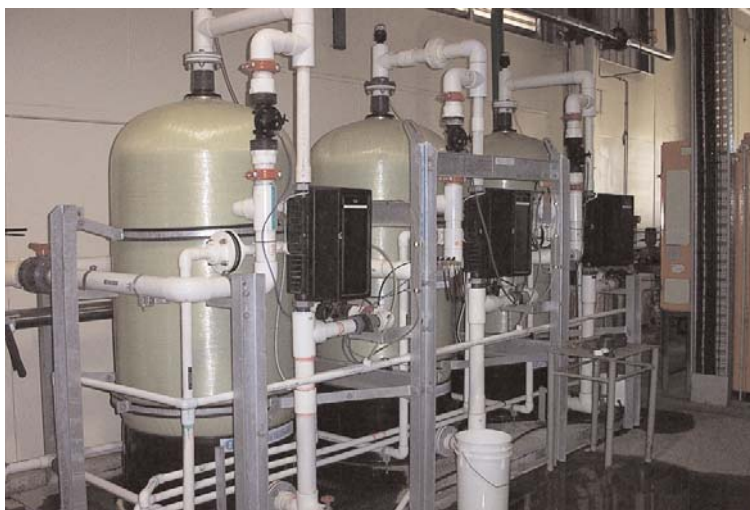
The treatment of boiler feedwater will help to minimise build-up of scale, which acts as an insulator and inhibits heat transfer.
