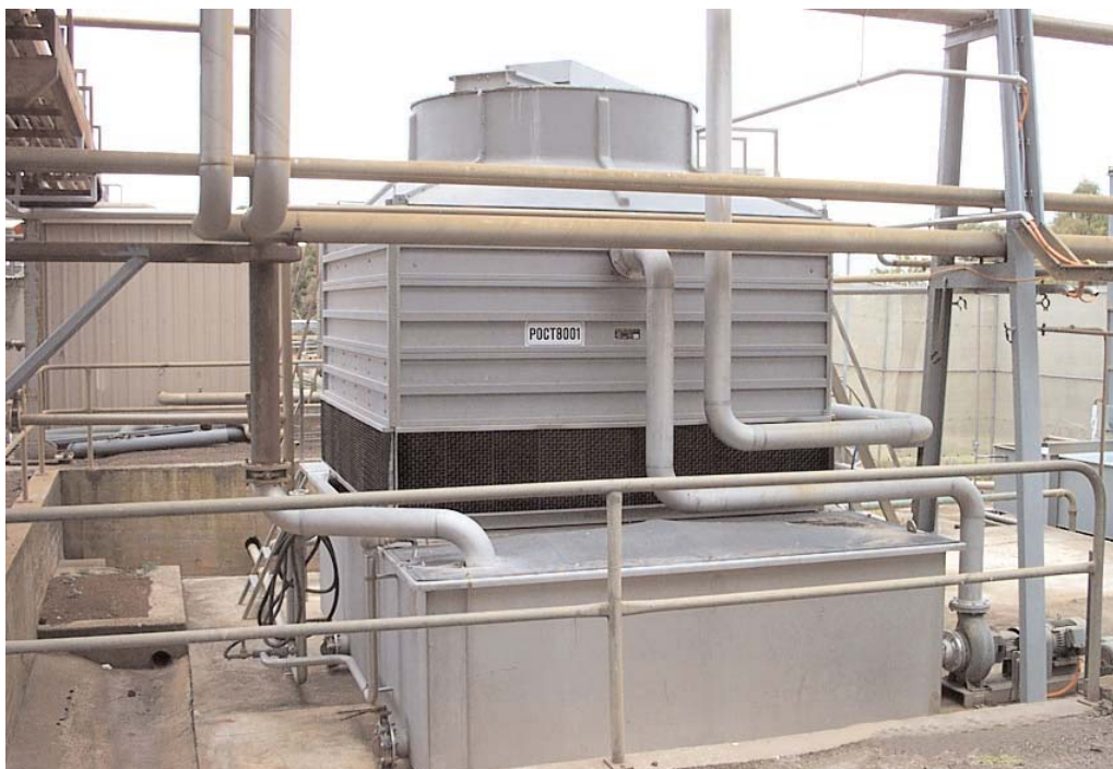
Cooling towers should be regularly checked for leaks and scale build-up.
