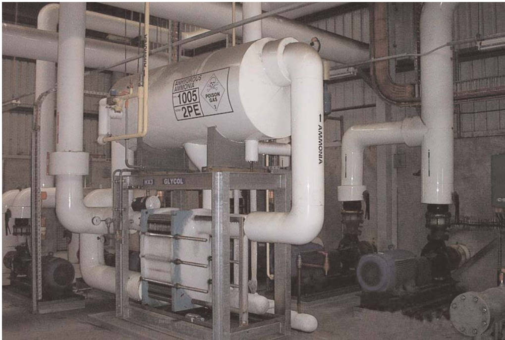
The cost of operating a refrigeration system can be up to around 20% of total energy costs in a dairy processing plant.
