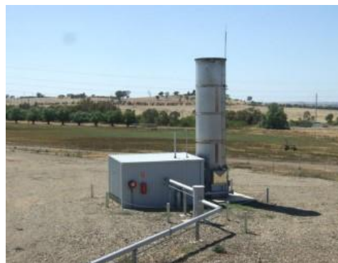
Image 6: Fully enclosed flare treating CAL biogas
