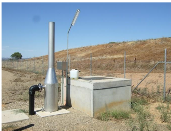
Image 10: Hydrostatic release valves
