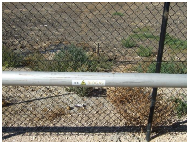
Image 13: Above ground stainless steel biogas pipe
