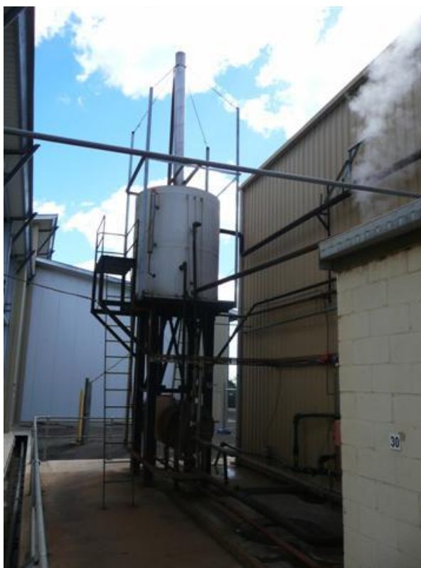
Photo: Plumes of flash steam from condensate tanks may be indicative of attractive heat and water recovery opportunities.
