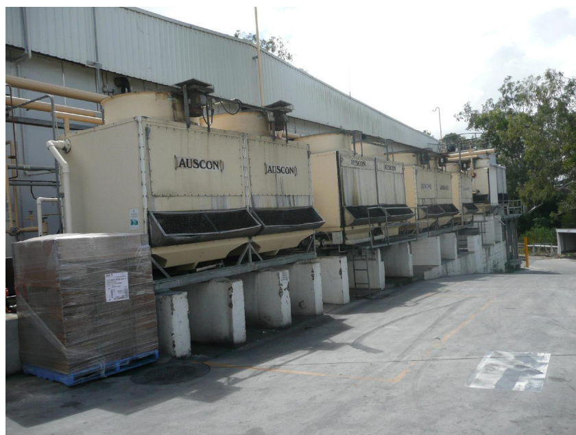
Photo: Condenser maintenance programs should ensure clean condenser surfaces, reduced spray water dispersion, and removal of non-condensable gases from the system
