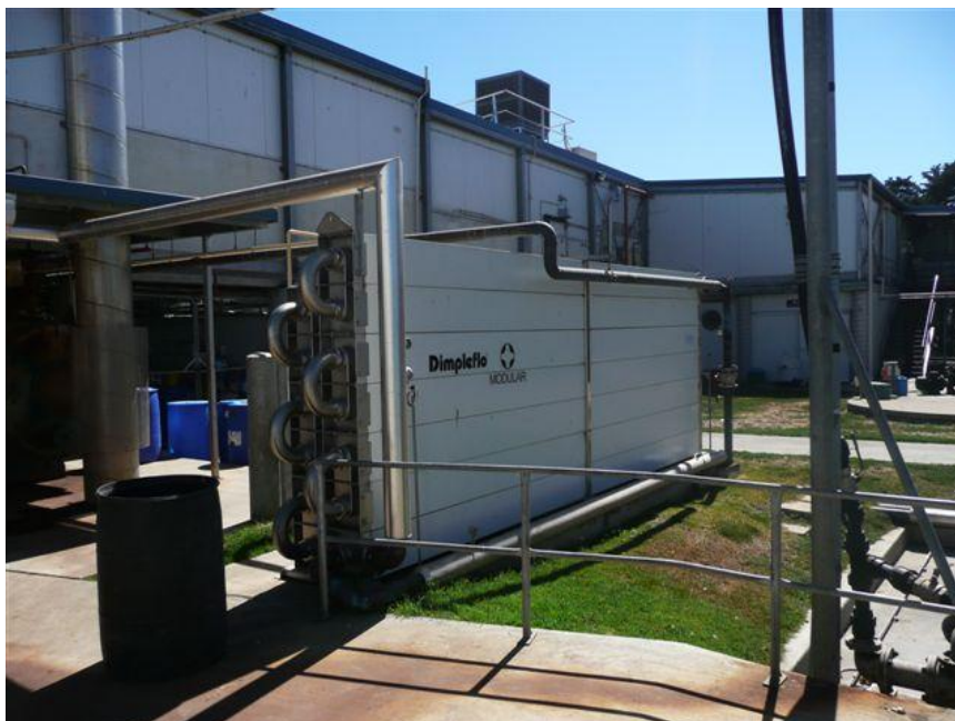
Photo: A heat exchanger preheating the incoming cold water with outgoing Sterilisers waste water
