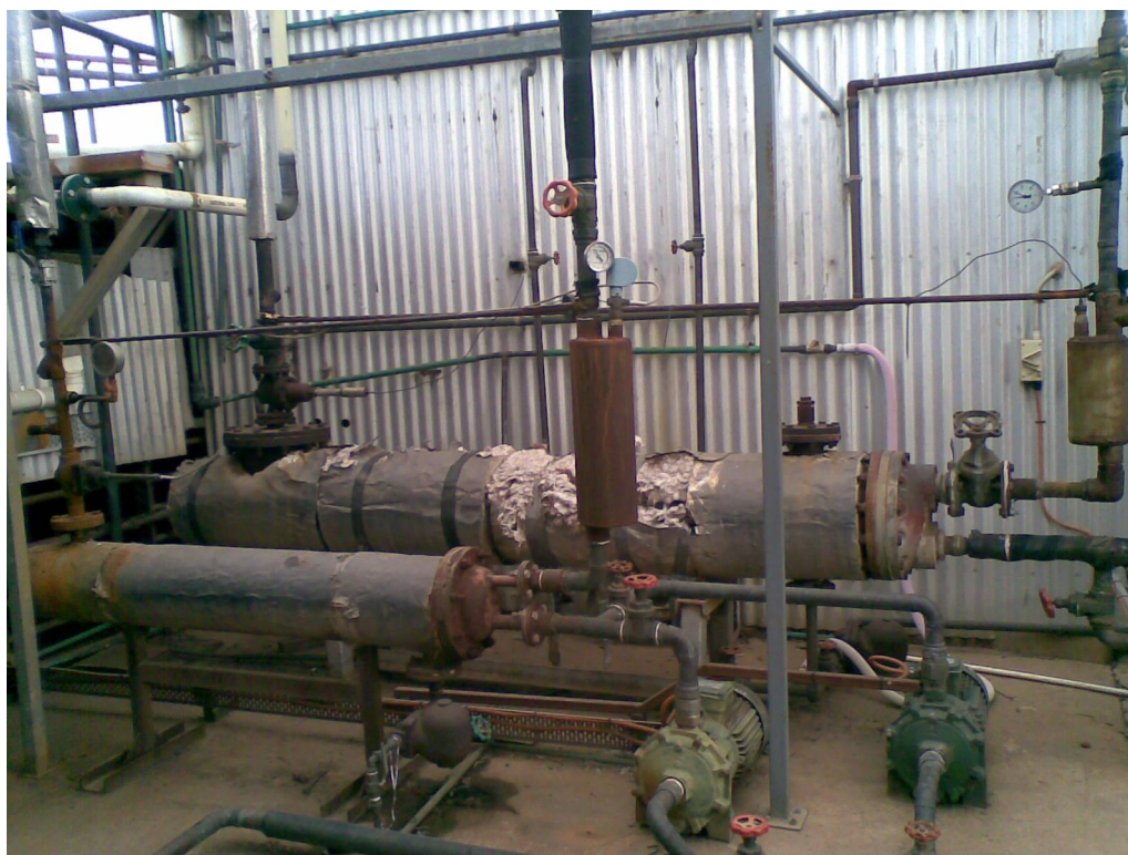
Photo: Locating heat exchangers close to the boiler house and repairing damaged insulation will reduce heat losses and fuel consumption.
