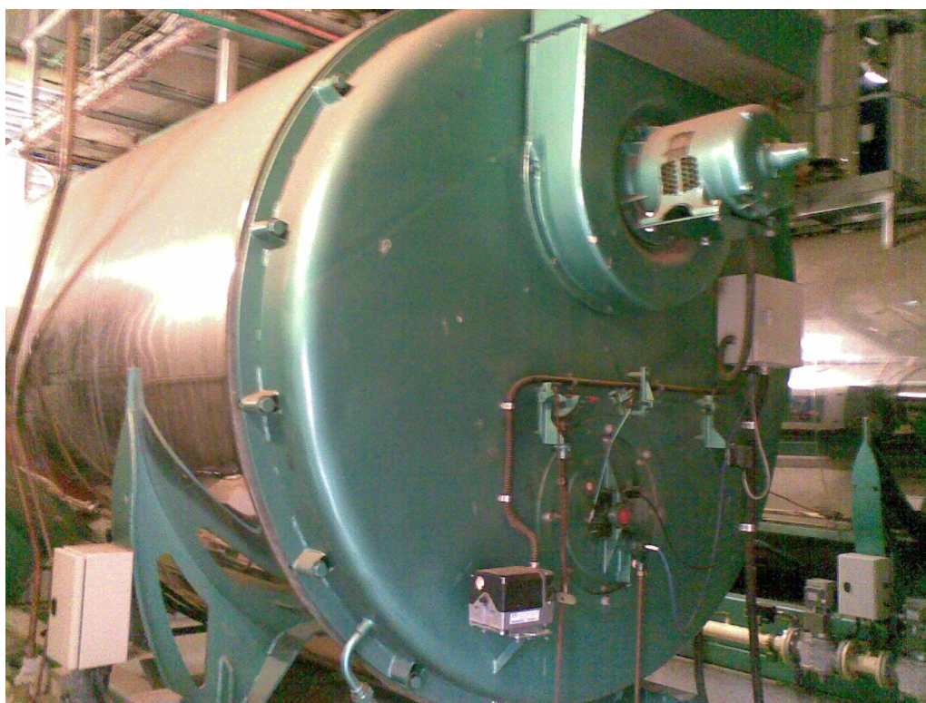
Photo: Regular combustion analysis and tuning of burners can ensure boiler operation at optimum combustion efficiency
