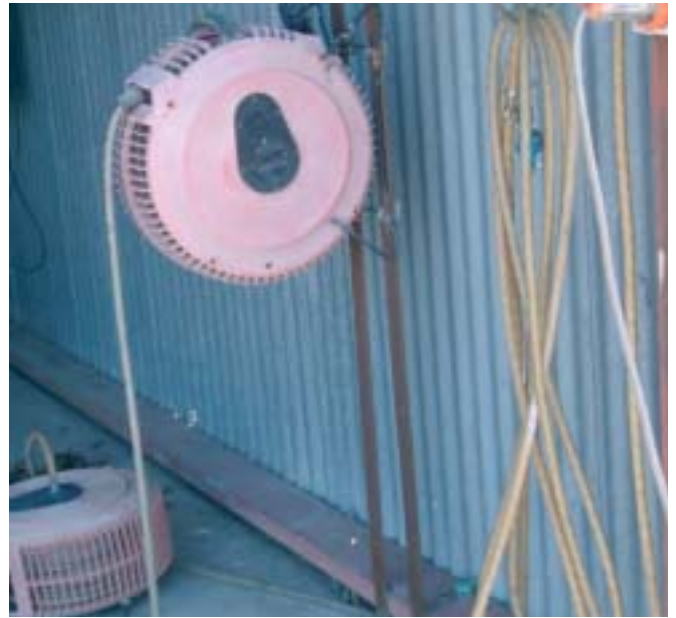
Compressed air ducted into the workshop
