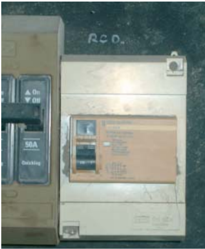
Residual Current Device fitted to circuit
