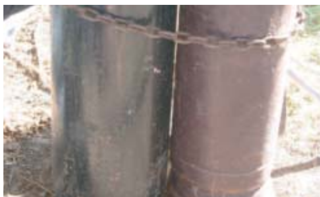
Oxyacetylene cylinders chained in position
