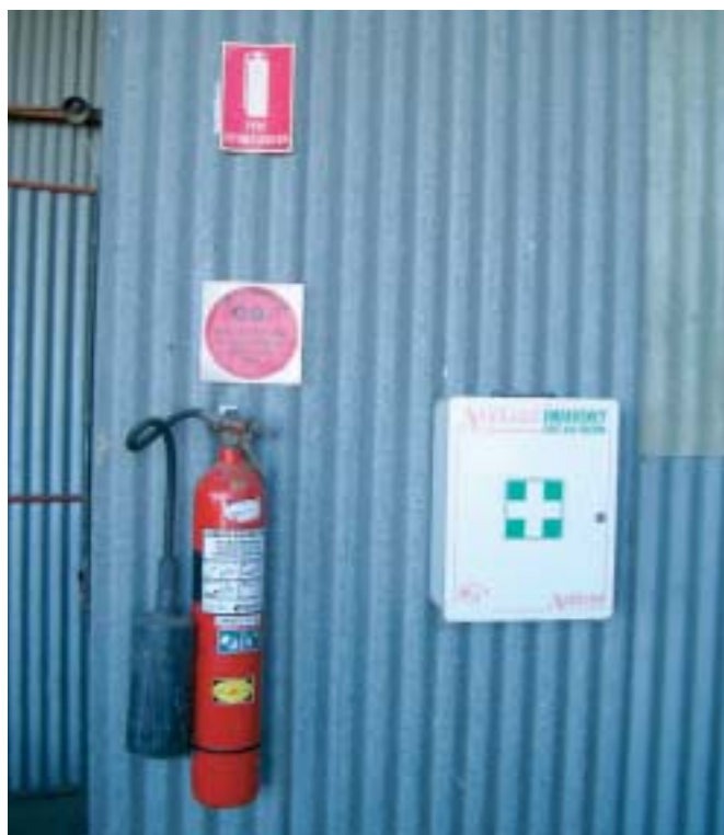
Clearly visible emergency equipment
