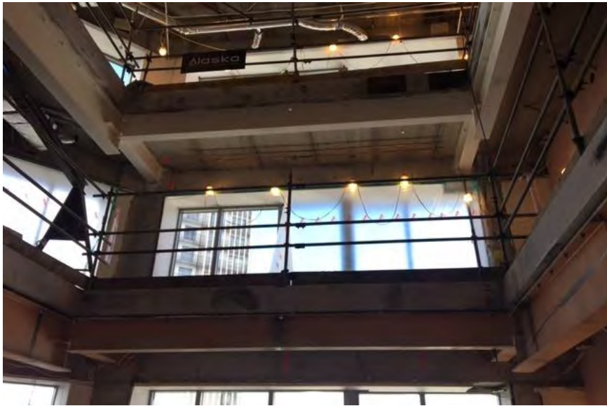
construction progress on Suncorp internal stair works between levels 11 and 15 (3 out of 4 floors completed)
