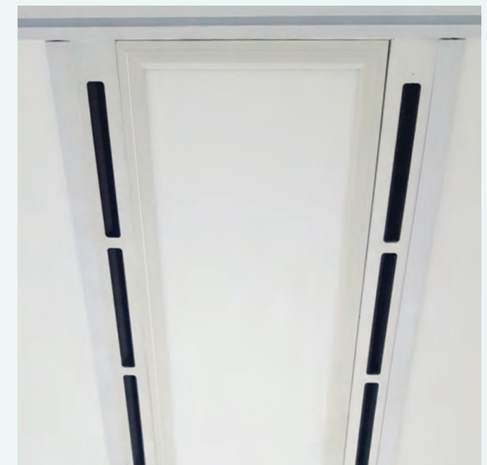
Custom retrofit LED panel
