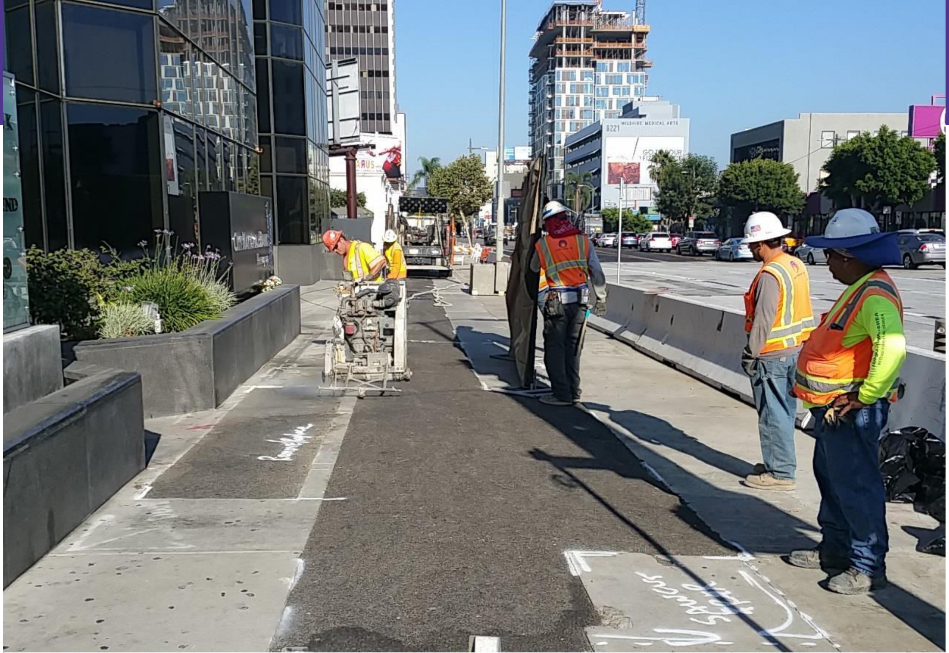
C1045 170808 832am STS Sawcutting for Concrete Sidewalk Restoration in front of 6100 Wilshire W of Fairfax facing W
