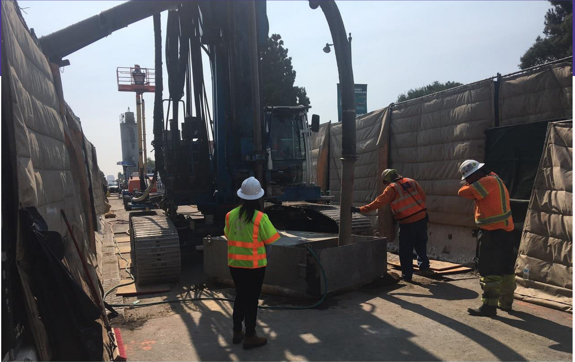
C1045.170712.958am.Metro Intern on site observing the Malcolm jet grout activities at Cross Passage 14 location looking E on Wilshire
