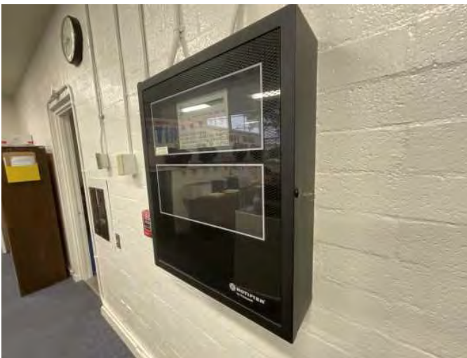
29 - FIRE ALARM PANEL
