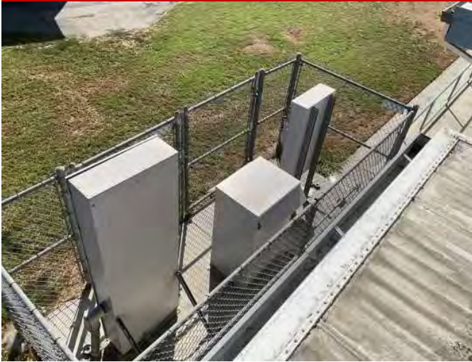
25 - MAIN ELETRICAL EQUIPMENT
