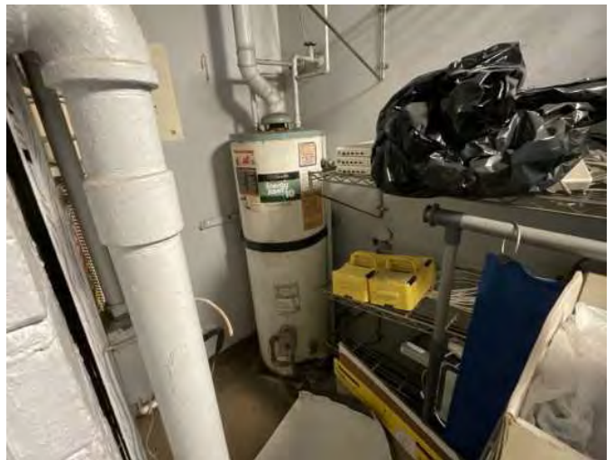
28 - DOMESTIC WATER HEATER
