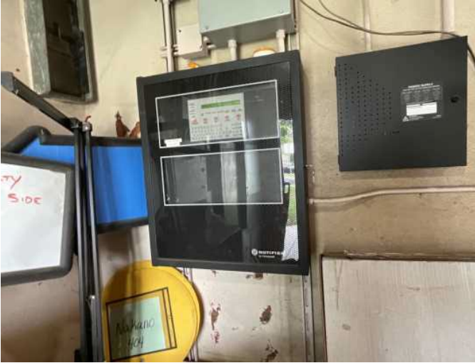
43 - FIRE ALARM PANEL
