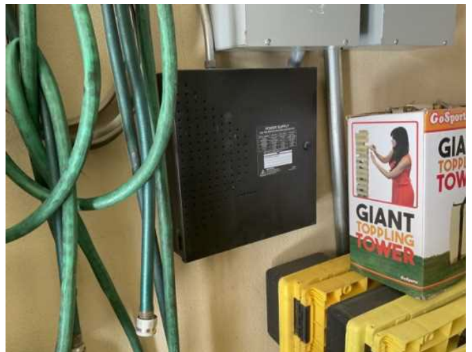
42 - FIRE ALARM PANEL
