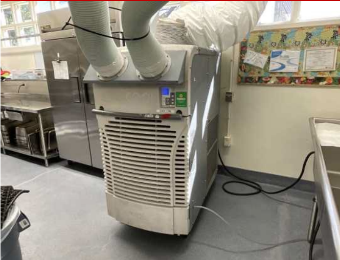
37 - KITCHEN AC UNIT
