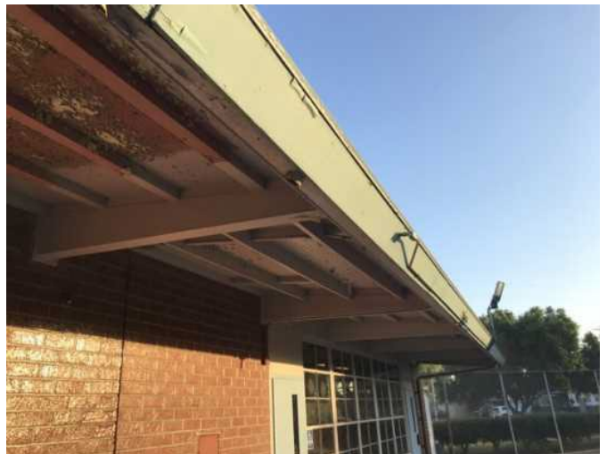
6 - DETERIORATED EXTERIOR FAÇADE
