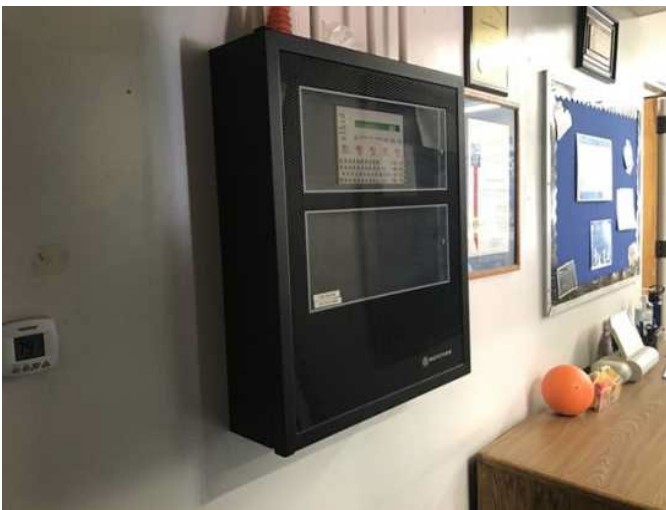
29 - FIRE ALARM PANEL
