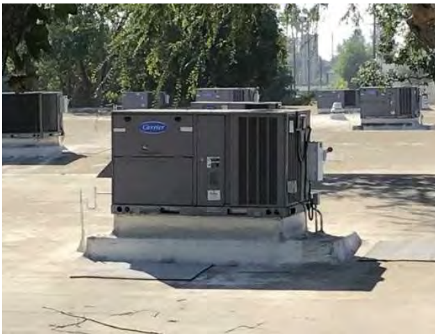
23 - PACKAGED UNITS (RTU)
