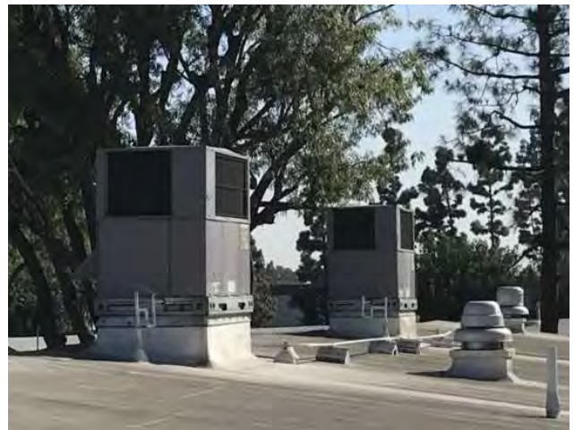
24 - PACKAGED UNITS RTU)
