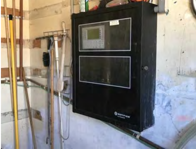
31 - FIRE ALARM PANEL
