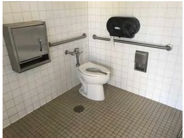
22 - TOILET, COMMERCIAL WATER CLOSET
