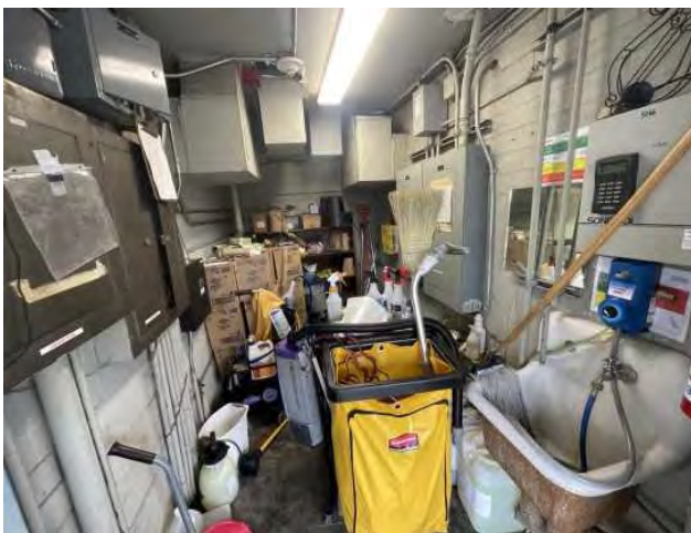
35 - TYPICAL ELECTRICAL ROOM
