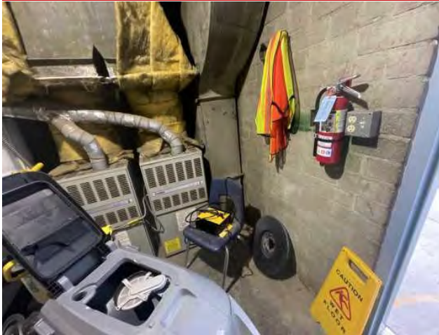
37 - MULTIPURPOSE BUILDING BOILER ROOM
