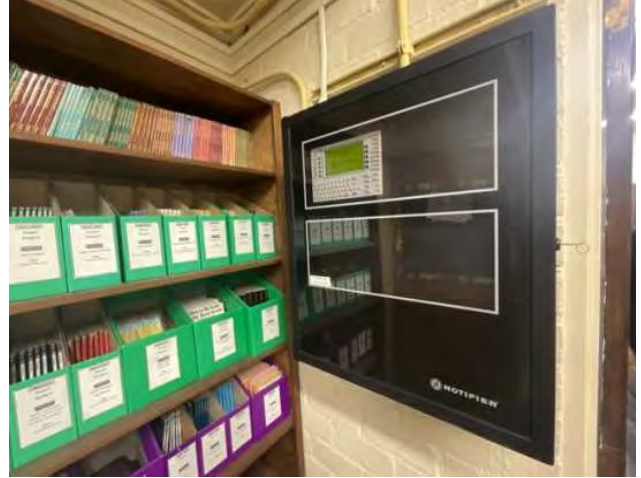
44 - FIRE ALARM PANEL
