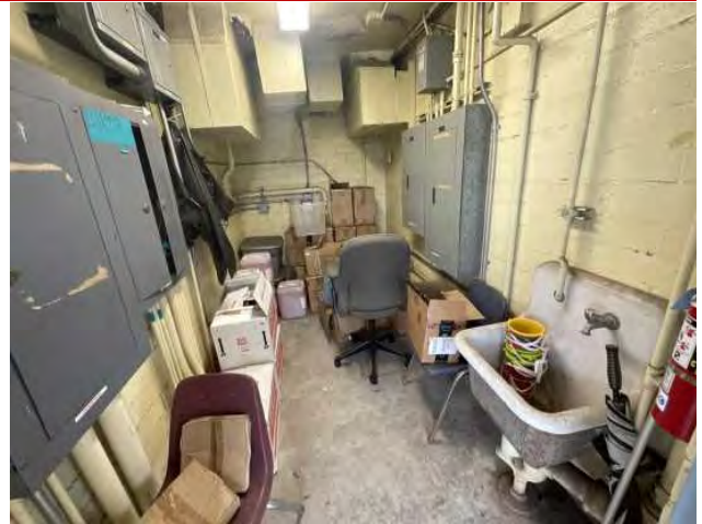
38 - TYPICAL ELECTRICAL ROOM
