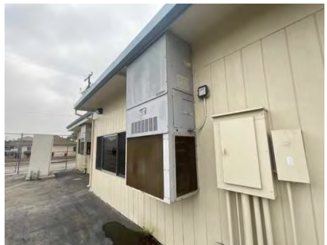
42 - HEAT PUMP - WALL-MOUNTED
