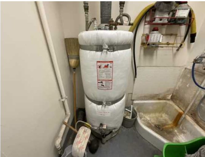
11 - MPR WATER HEATER
