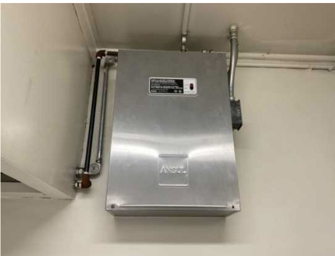
17 - FIRE SUPPRESSION SYSTEM
