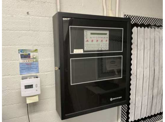
20 - FIRE ALARM PANEL
