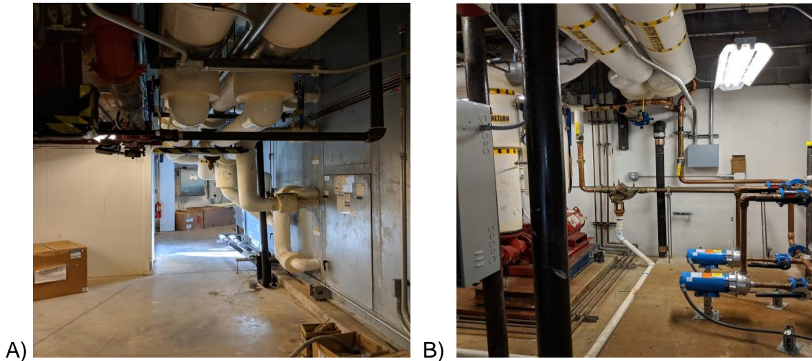
Figure 4-2. Mechanical Room, Rinker Hall A) West facing and Figure B) East facing (Source: Courtesy of the author, 2018)
