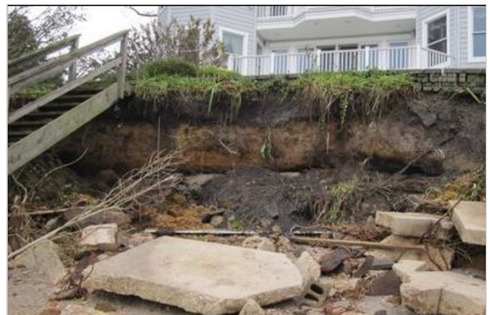
Damage caused by Sandy in October 2012
