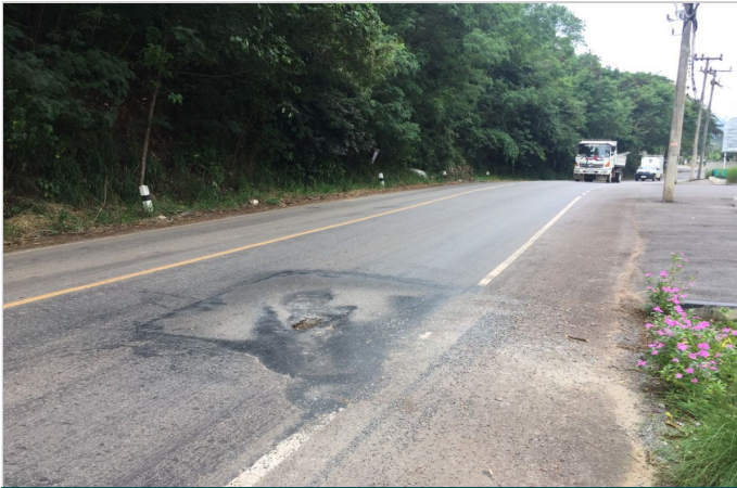
Damaged Pavement Due to Rockfall Debris Impact
