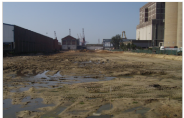
The top 1.5m of in situ material was removed in readiness of the contraction of
