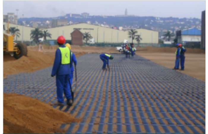
The next layer of compacted decomposed granite was laid on top of the first layer
