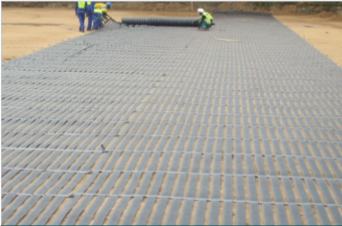
A compacted layer of decomposed granite was placed on top of the geotextile foil
