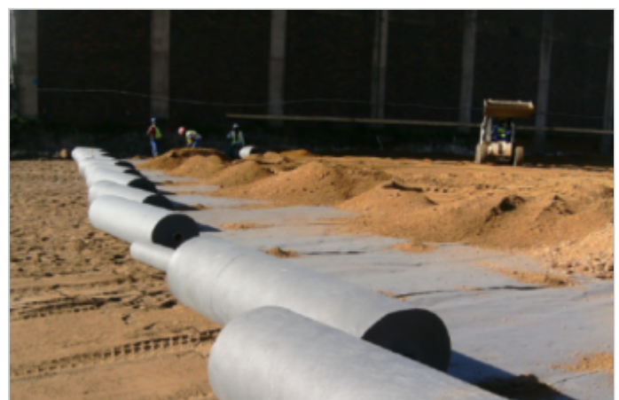
A Layer of the river sand sandwiched between two layers of AG 400 geotextile pro
