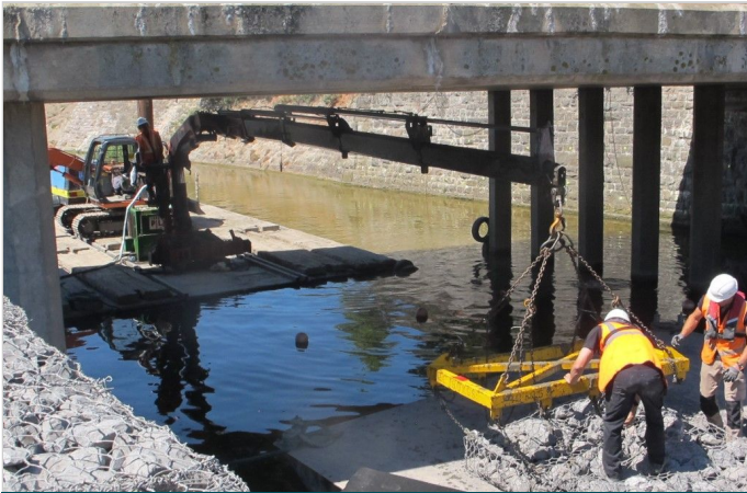
Prefilled gabion on the pontoon ready to be placed on the channel bed
