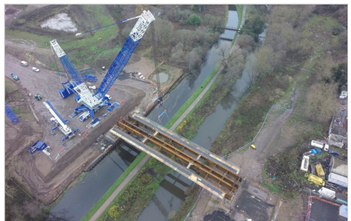
Crane outriggers/pads placed very close to the front face of the reinforcement.
