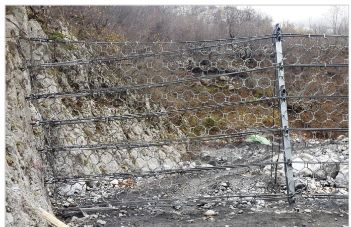
Debris Flow Barrier 200 KJ after installation
