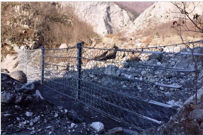
Debris Flow Barrier 200 KJ after installation
