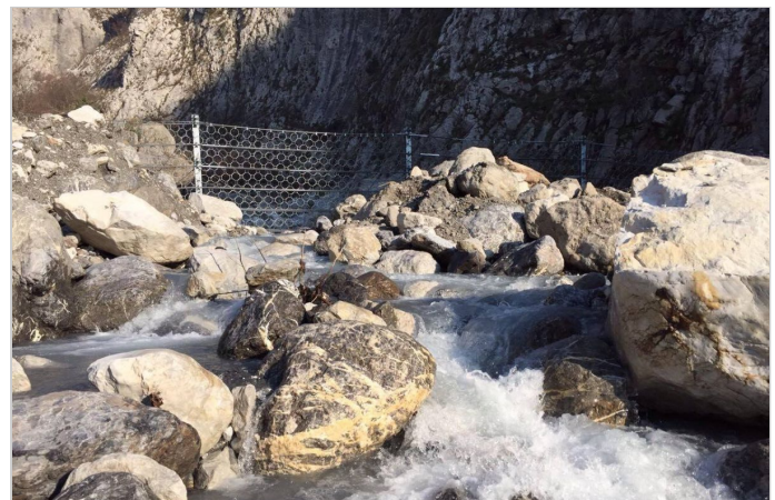
Debris Flow Barrier 200 KJ after installation
