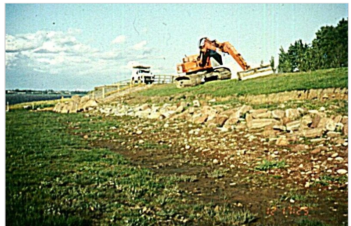
Existing scour line
