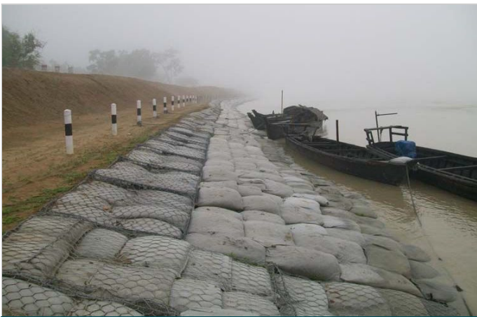
Photo 5: Condition of MacBag® and river bank after flood
