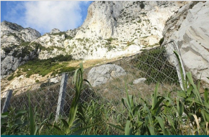
View of slope from the road showing boulders
