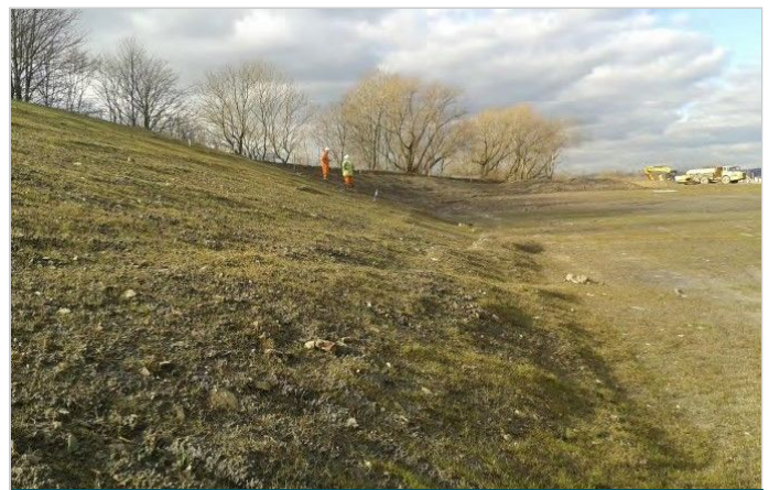
Bulging and tension cracks of the face slope in Winter 2016
