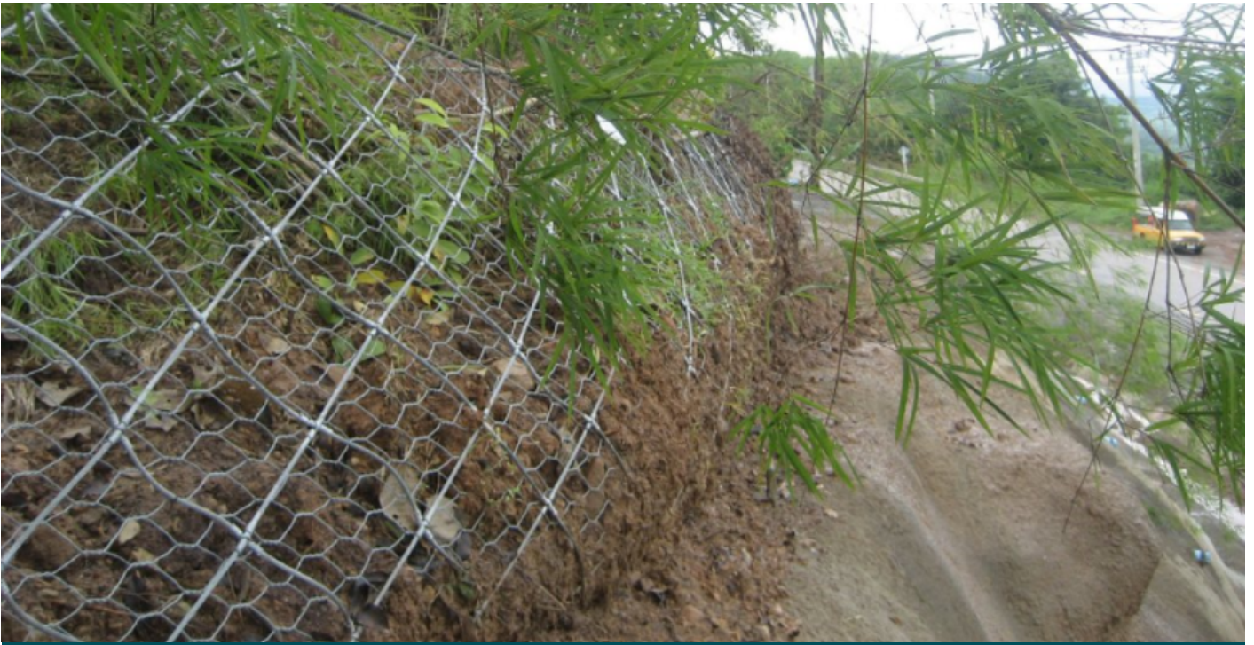
Debris Flow Barrier After Impact
