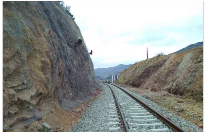
Rockfall Protection System
