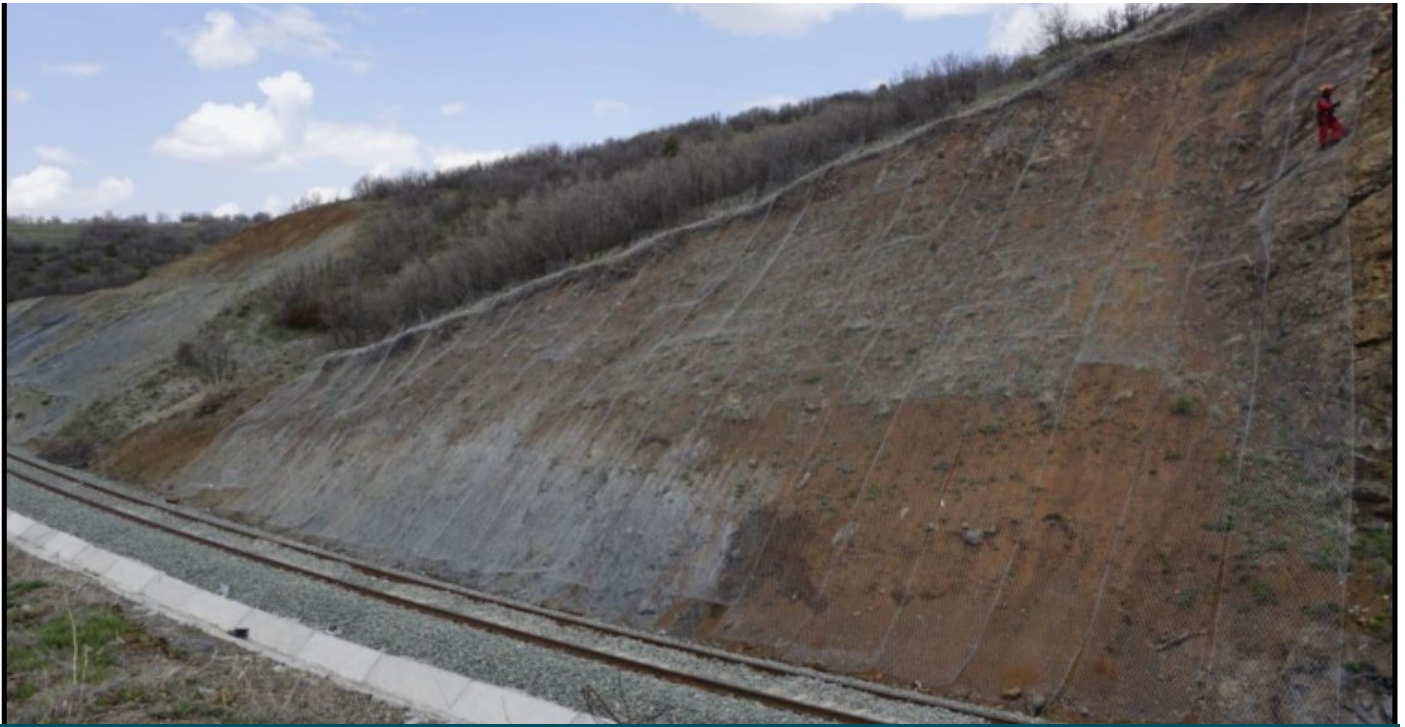
Rockfall Protection System
