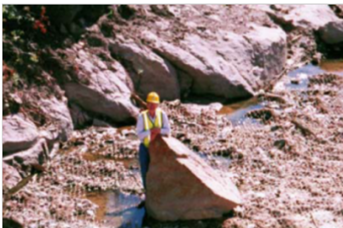
Example of debris (on top of Gabion Mat®) following storm
