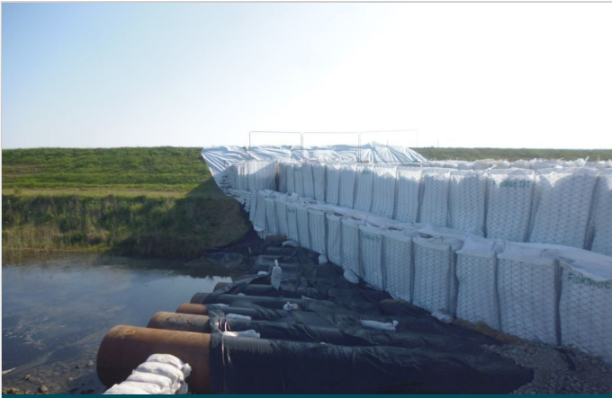
FlexMac units crossing drainage tubes
