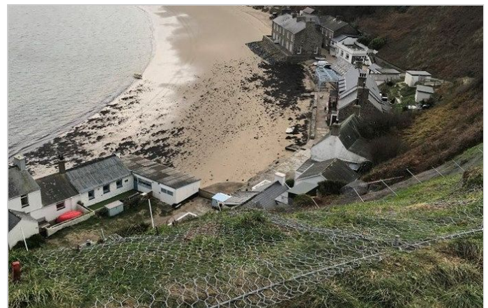
DT rockfall netting secured around a crest rope
