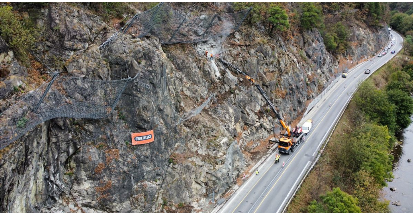
General elevation view on rockfall protection
