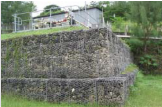
Corner view of wall post earthquake
