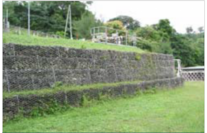
Front view of wall post earthquake
