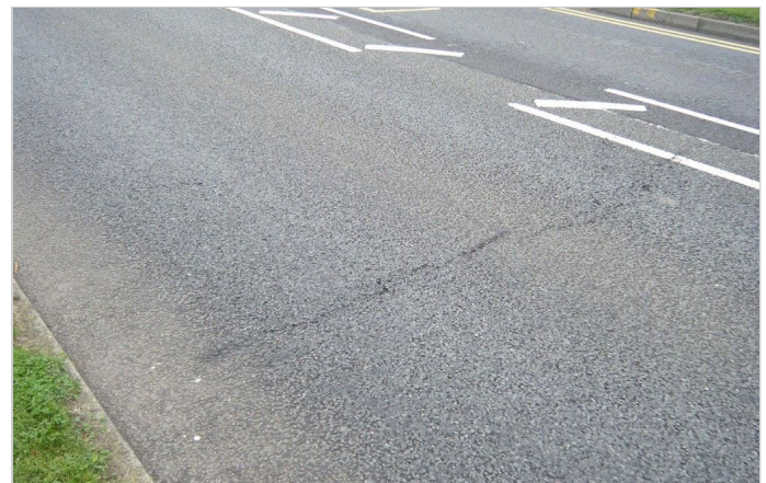
Transverse cracking apparent on unreinforced section
