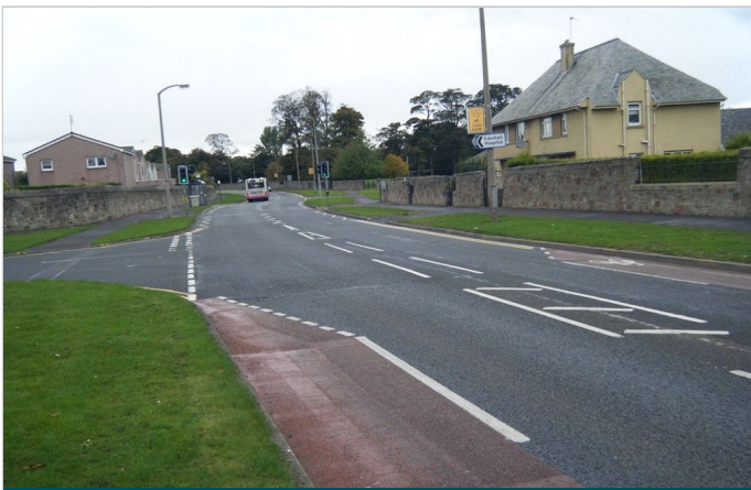
Prior to overlay, the pavement required constant maintenance
