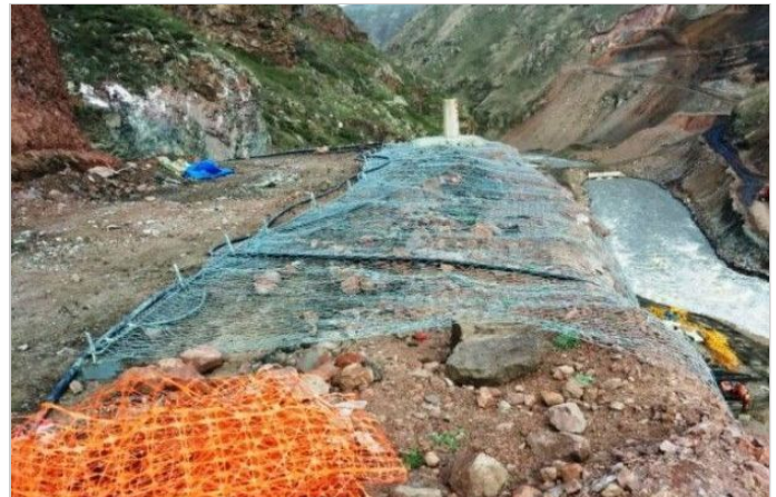
Rockfall Protection at Ardahan Dam
