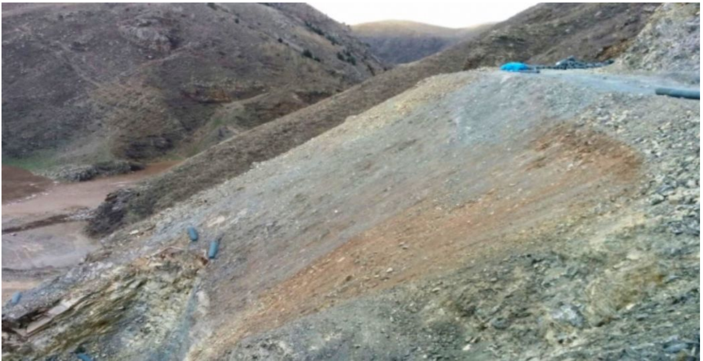
Rockfall Protection at Ardahan Dam
