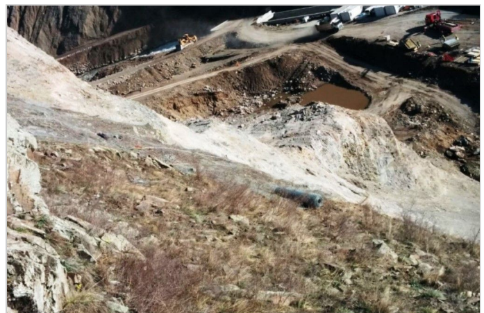
Rockfall Protection at Ardahan Dam
