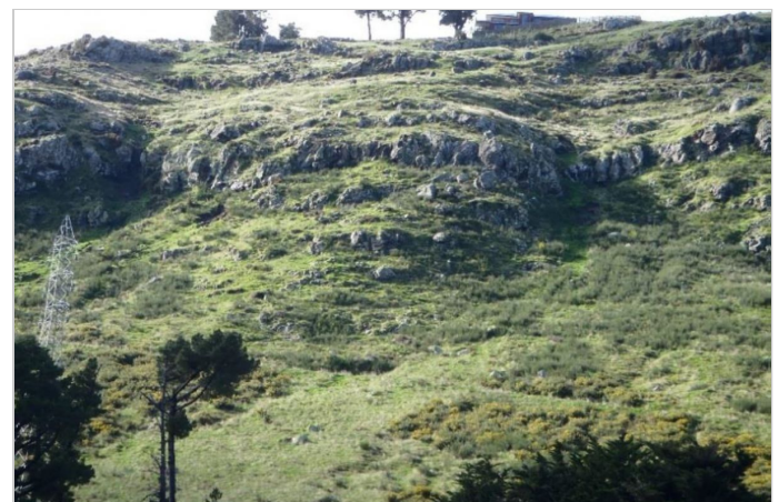
Photo showing multiple rockfall points upslope of pylon
