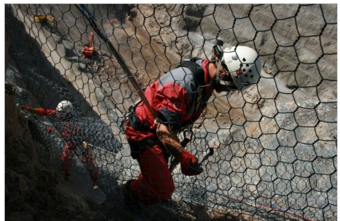
Rockfall protection at the Highdam site
