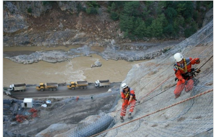
Rockfall protection at the Hydroelectric Power Plant site
