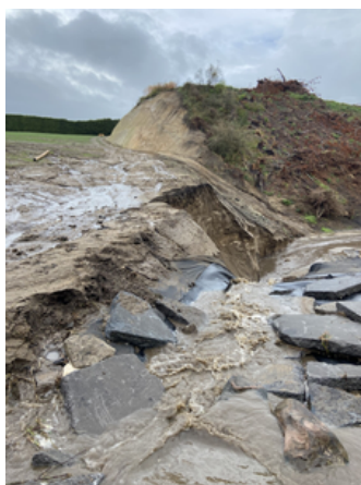
Left: Compliance Officer collecting sediment-laden water samples from the failed spillway for analysis. Right: Failed spillway associated with the newly contoured site highlighting poor construction.
