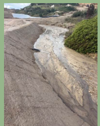
Photos: showing short length which will cause erosion and long tail causing blockage
