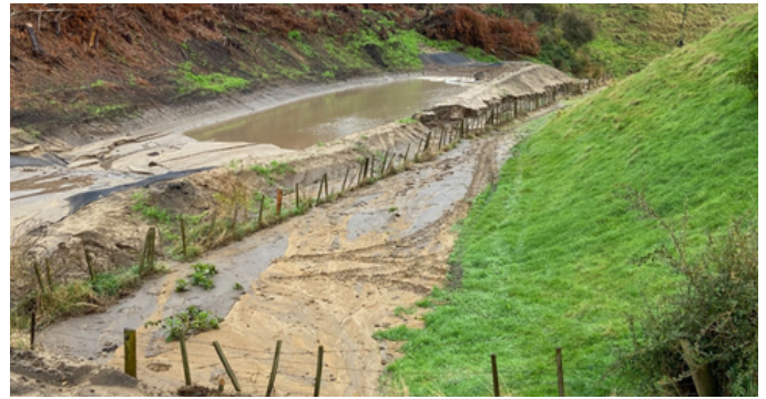
Remains of the poorly constructed sediment retention pond following failure.
