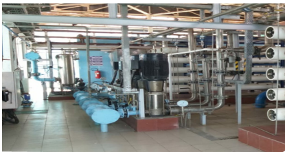
District Cooling Plant
