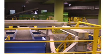
Automated Waste Collection & Segregation Plant
