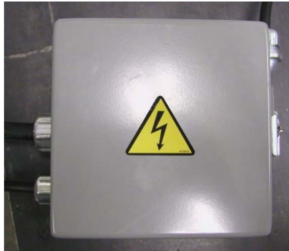
MAGNET RELAY KIT AS INSTALLED
