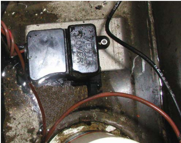
FLOAT SWITCH AS INSTALLED IN BWC-2
