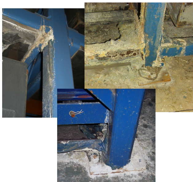
Corrosion damage due to improper drip pan maintenance
