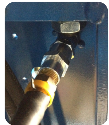
In-line filter mounted on BE vacuum
