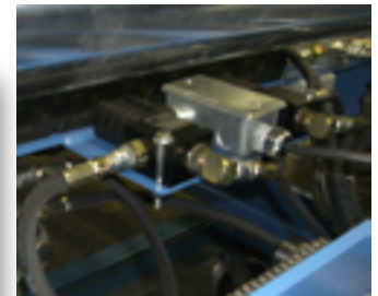
Solenoid valves mounted in center compartment under extractor arm.
