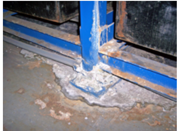
Corrosion damage to stand and floor due to poor drip pan maintenance
