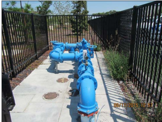
8-INCH CALWATER INTERTIE INDUSTRIAL RD (PAMF)
