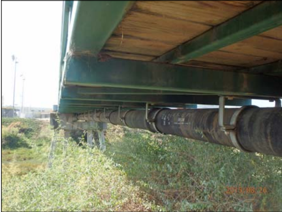
12-INCH DIP SUSPENDED UNDER PEDESTRIAN WALKWAY O'NEILL SLOUGH SPORTS FOOTBRIDGE
