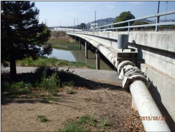
12-INCH DIP SUSPENDED ALONG BRIDGE ISLAND PARKWAY BRIDGE
