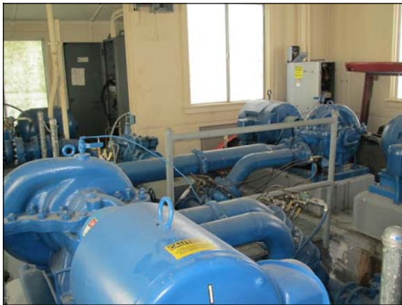
INTERIOR OF FOLGER PUMP STATION
