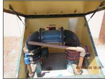
6-INCH CALWATER INTERTIE NORTH RD
