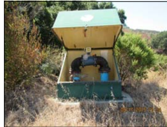
6-INCH CALWATER INTERTIE WITHERIDGE AVE
