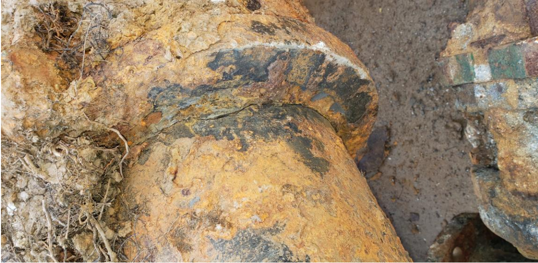
(externally - the ring break is visible where the Tee and Pipe meet)
