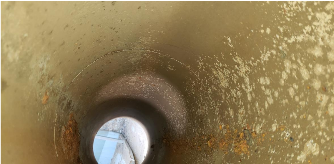
(internally – the ring break of the 10” pipe is visible covering about 2/3 of circumference)
