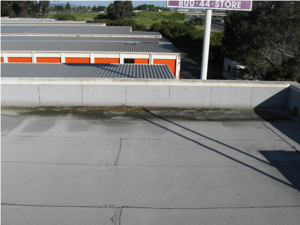
Photo 8: Typical Water Ponding on Roof
