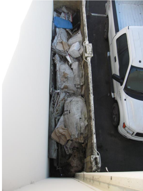
Photo 14: Excessive Amounts of Garbage Storage against Building
