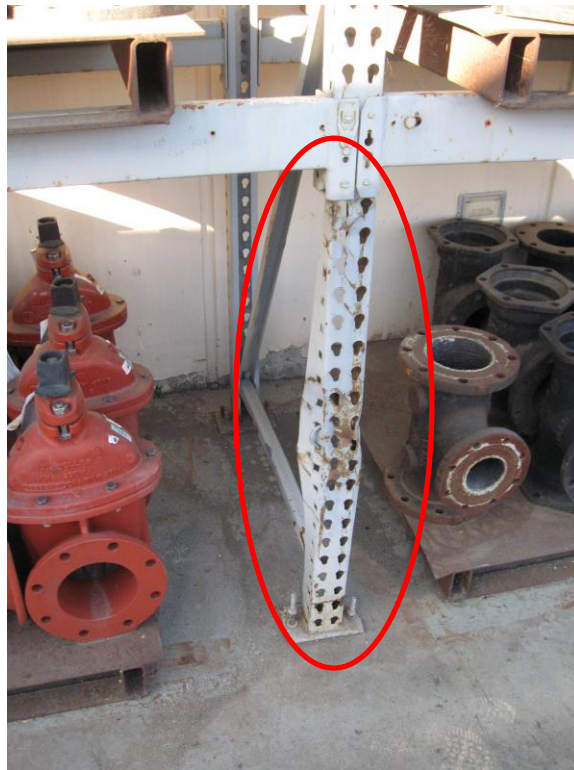
Photo 11: Minor Damage to Storage Rack Post & Loose Anchor Bolt Nuts
