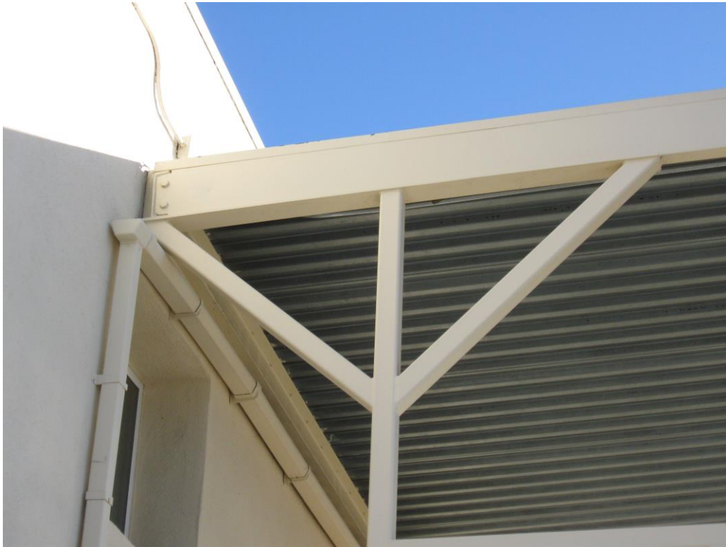
Photo 21: Insufficient Connection to Building
