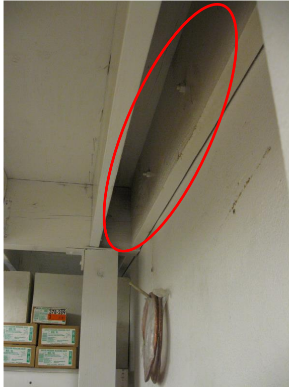
Photo 16: Typical Inadequate (Cross-Grain Bending) Mezzanine Floor to Wall Attachment
