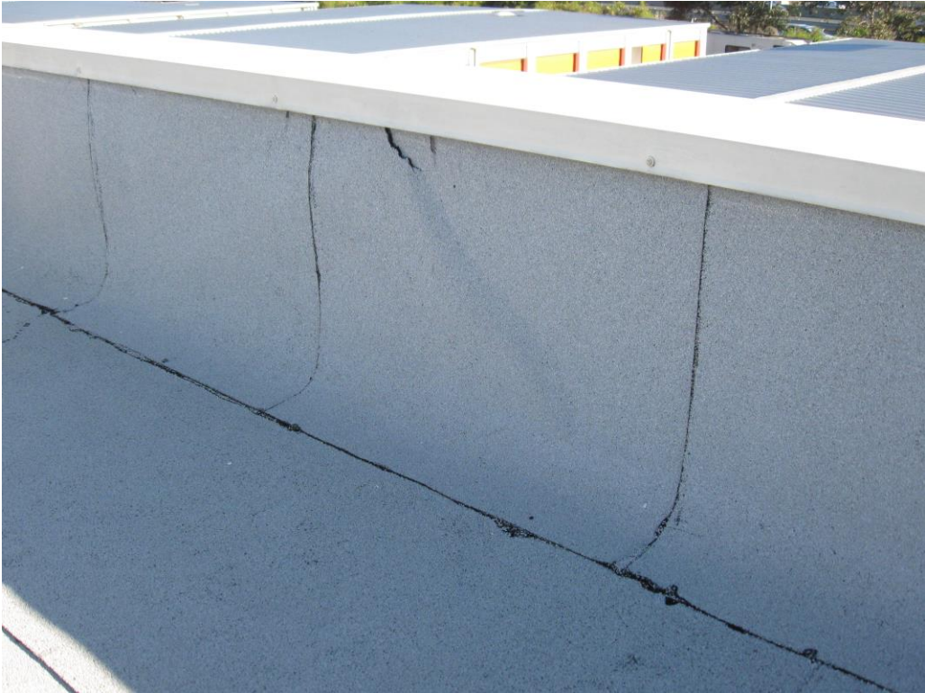
Photo 9: Typical Cracks and Bubbles in Roofing at Parapets
