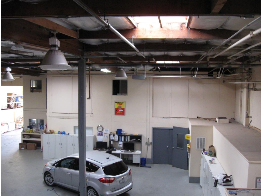
Photo 23: Typical Interior Mezzanine with Inadequate Lateral System
