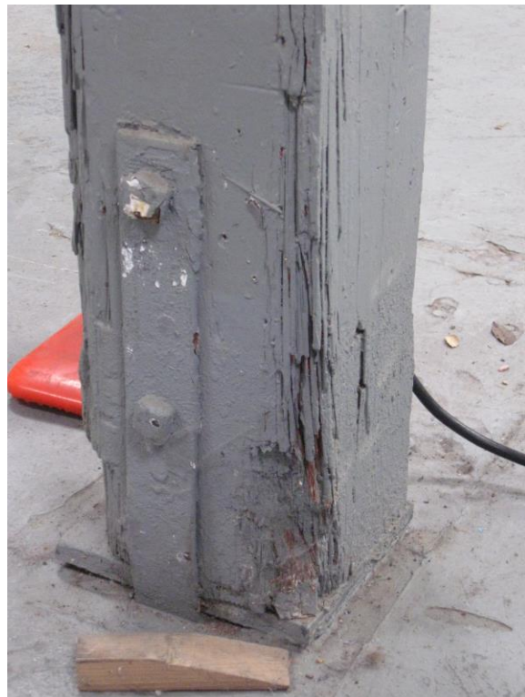
Photo 15: Minor Damage to Interior Wood Post
