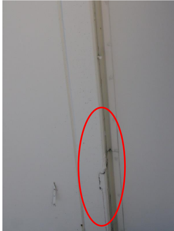
Photo 19: Cracked Concrete Pilaster at Seismic Joint
