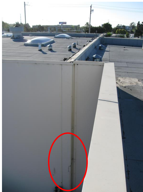
Photo 18: Cracked Concrete Pilaster at Seismic Joint
