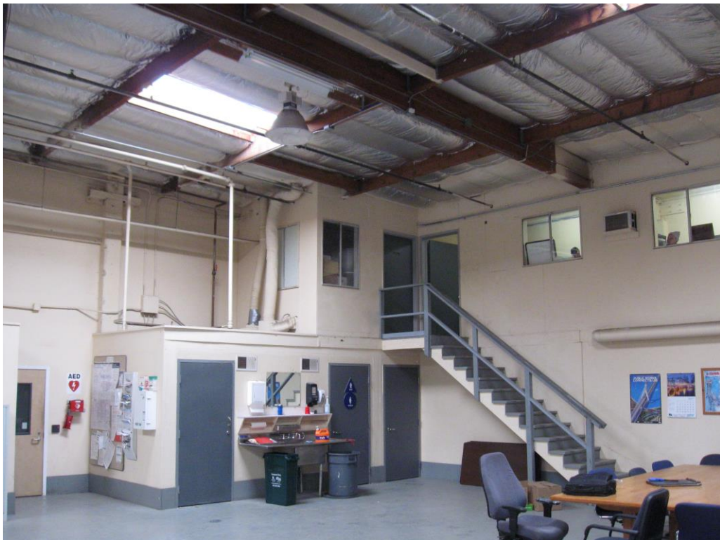
Photo 22: Typical Interior Mezzanine with Inadequate Lateral System
