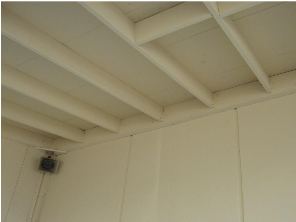
Photo 4: Inadequate Ledger Connection
