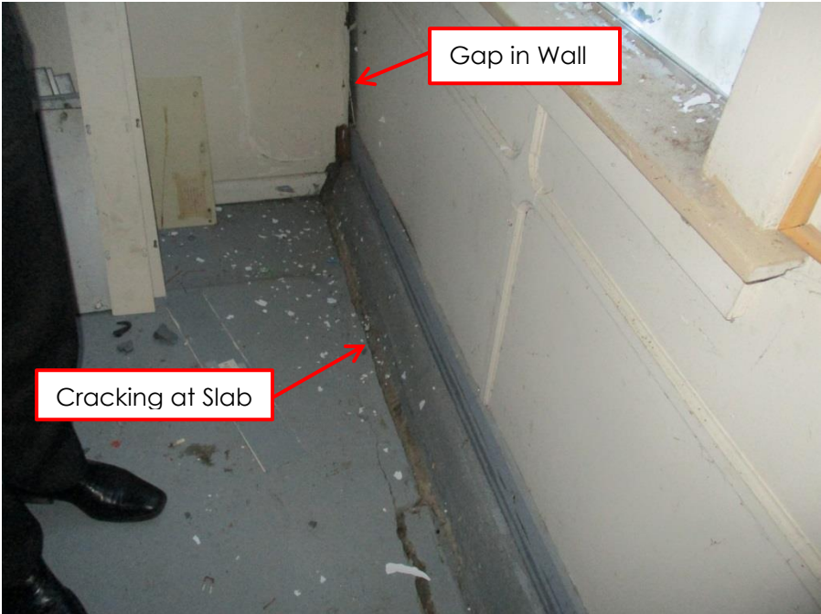
Photo 4: Cracking at Concrete Curb to Slab-On-Grade Interface and Gap in Wall
