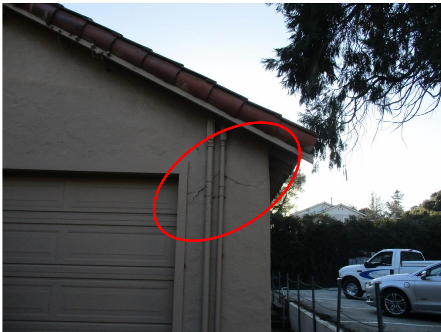
Photo 6: Cracks in Wall Adjacent to Garage Door
