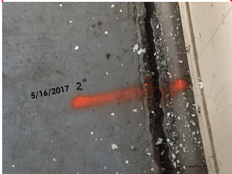
Photos 13 and 14: Measured Crack Width at Slab-on-Grade
