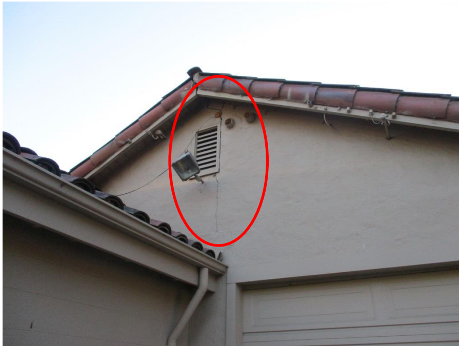
Photo 5: Cracks in Wall At Louver
