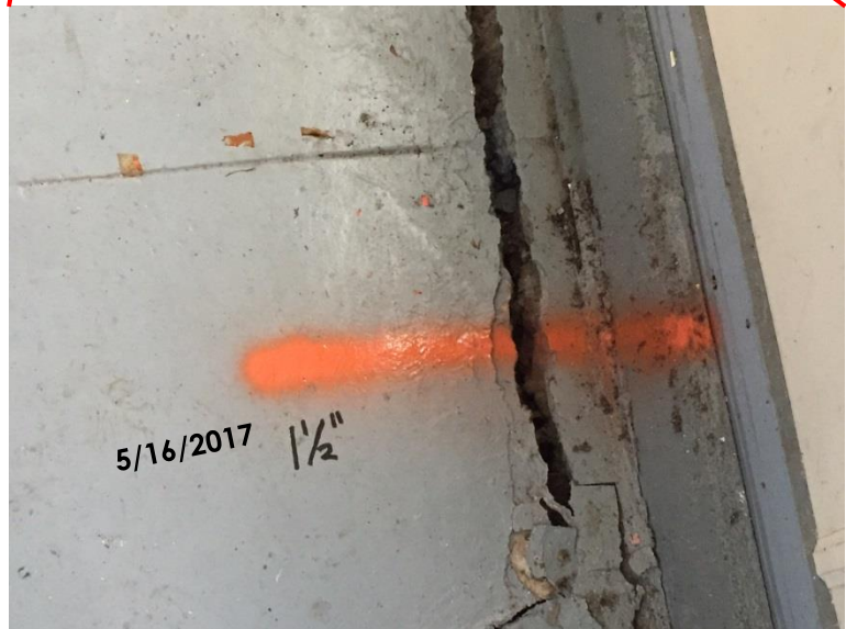
Photos 11 and 12: Measured Crack Width at Slab-on-Grade
