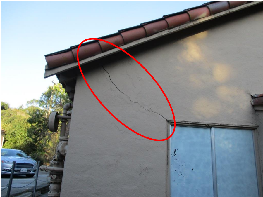
Photo 7: Cracks in Wall At Window Header
