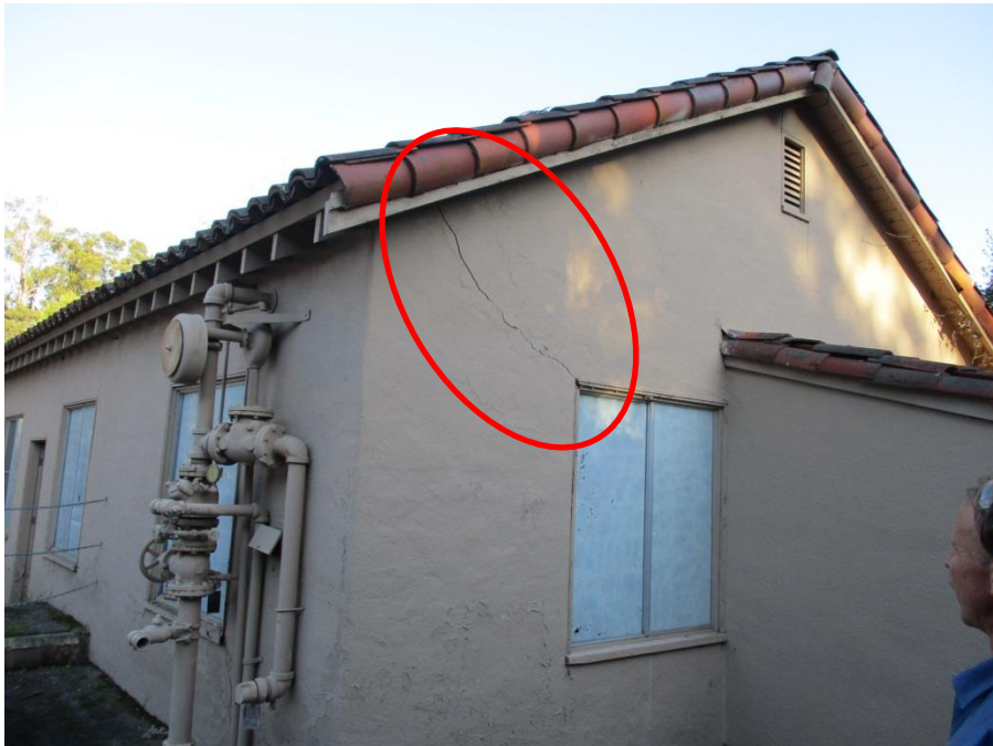
Photo 8: Cracks in Wall at Window Header
