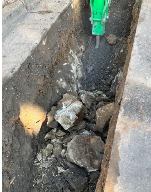
April 25, 2022 – Hoe ram used to break rock within trench on Vine St.
