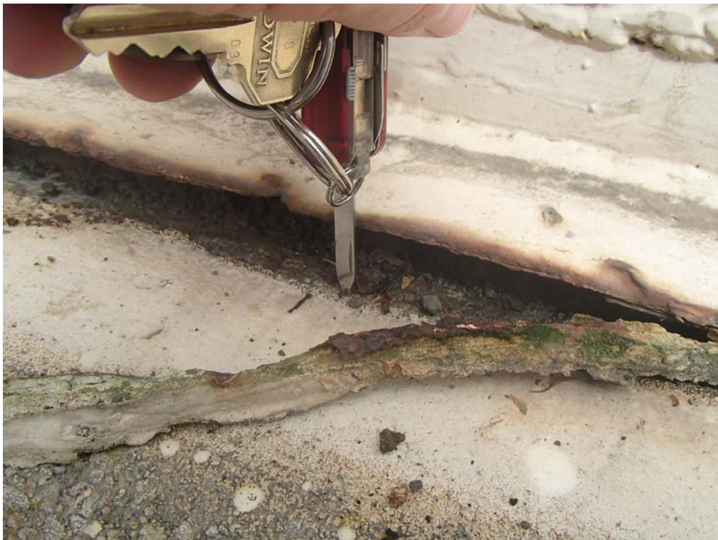
Photo 10: Degraded Caulking along Perimeter of Tank Bottom Plate
