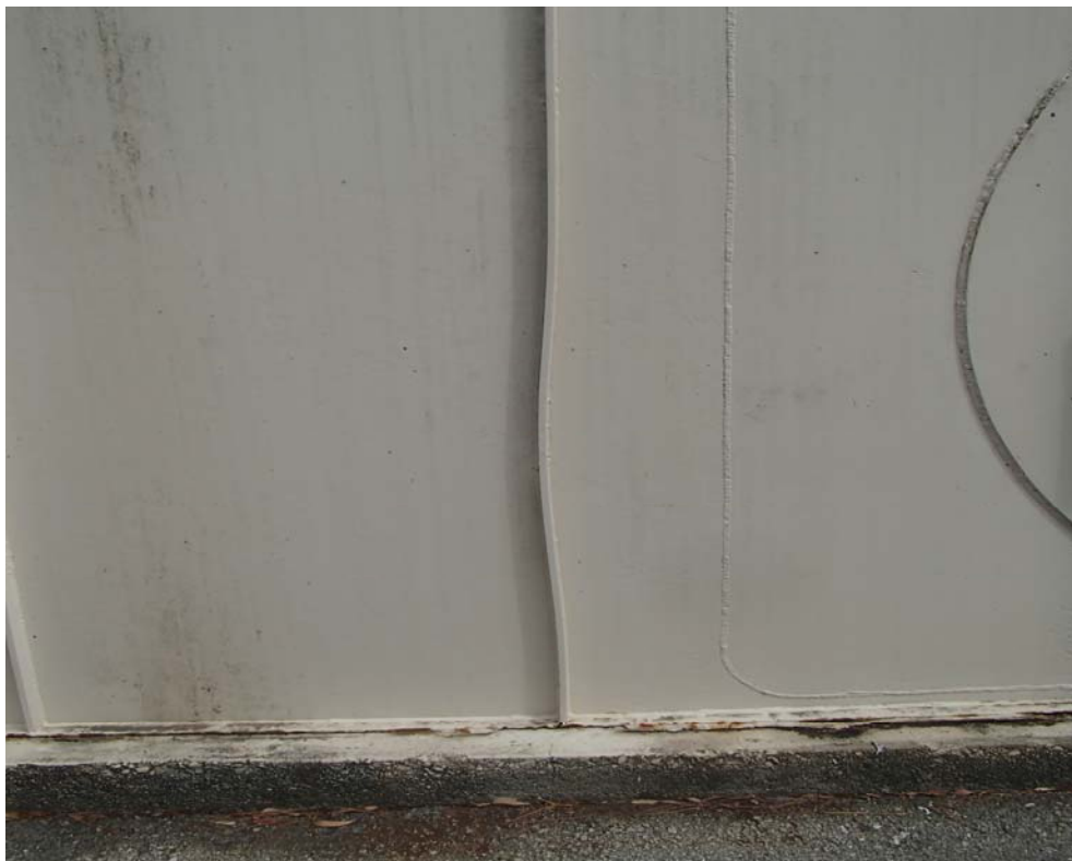
Photo 4: Misaligned Tank Stiffener Plate
