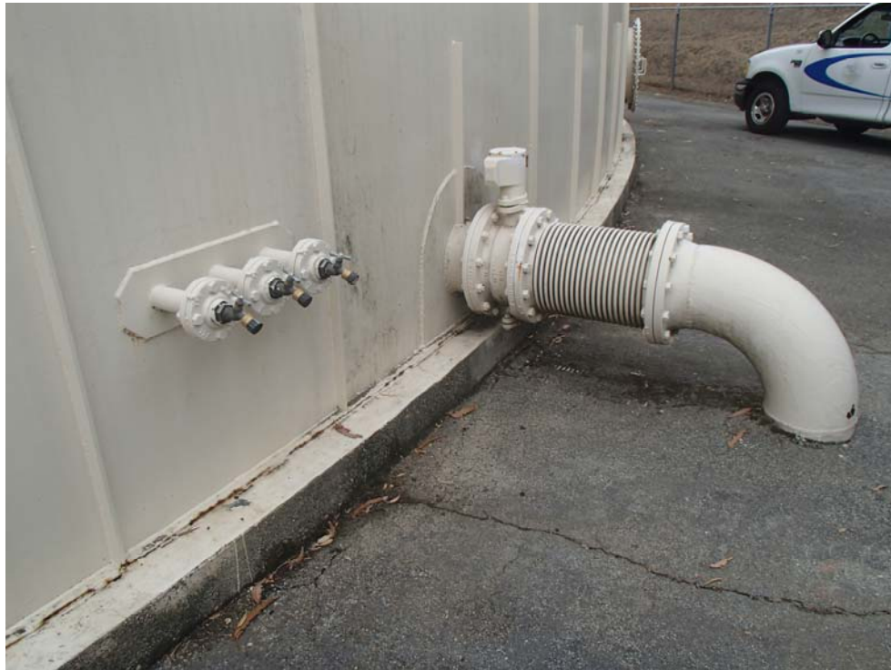
Photo 3: Inlet/Outlet Pipe with Flexible Connection
