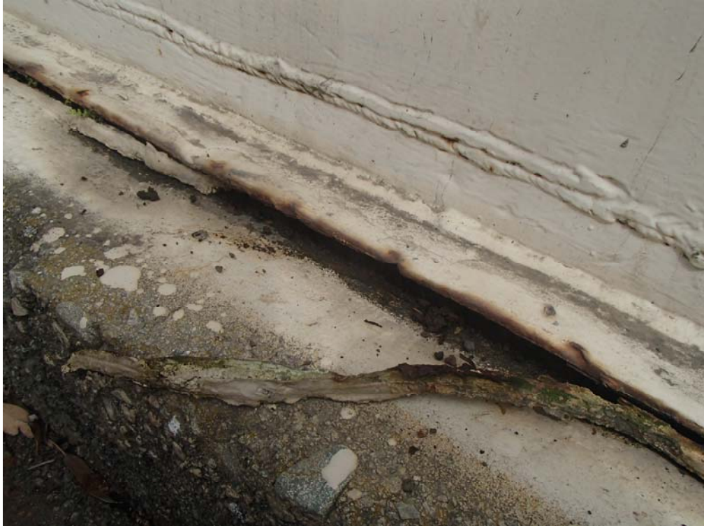
Photo 9: Corroding Tank Bottom Plate
