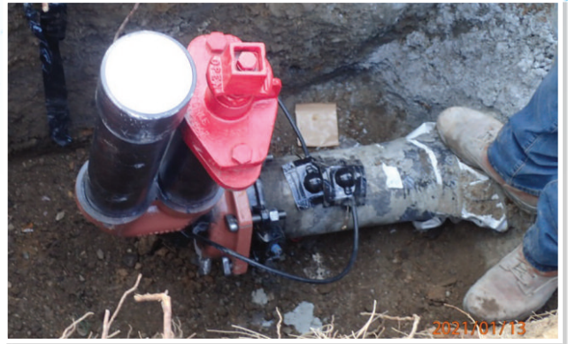
Above: The 4-inch blow off assembly at the end of the new water main at the SR101 Crossing at Palo Alto Medical Foundation (PAMF) site.
